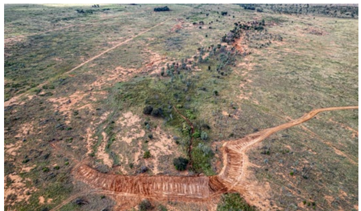
Above Right. Scaled areas are ripped on the contour to slow water velocity and allow the water to infiltrate to allow the natural grasses to recover and halt the gully erosion.
