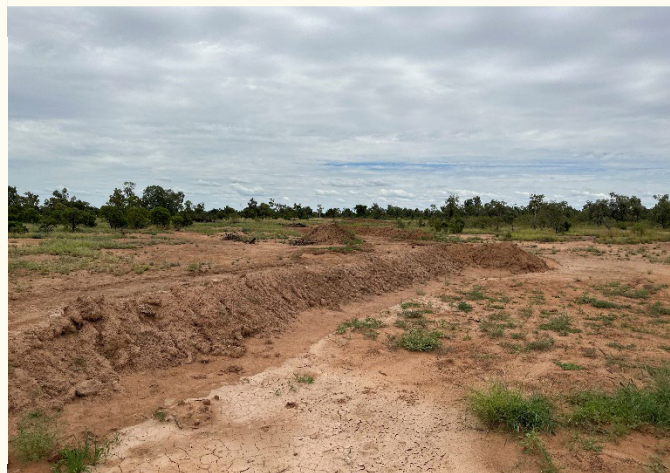
Spreader banks designed to divert water from a gully over a large flat area.
