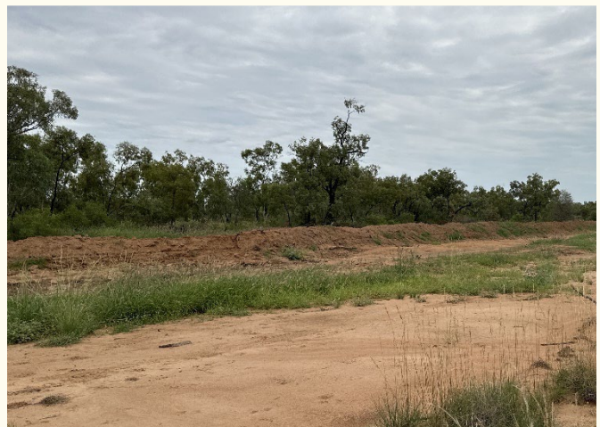
Earthen bank designed to divert water from a gully into a series of spreader banks.
